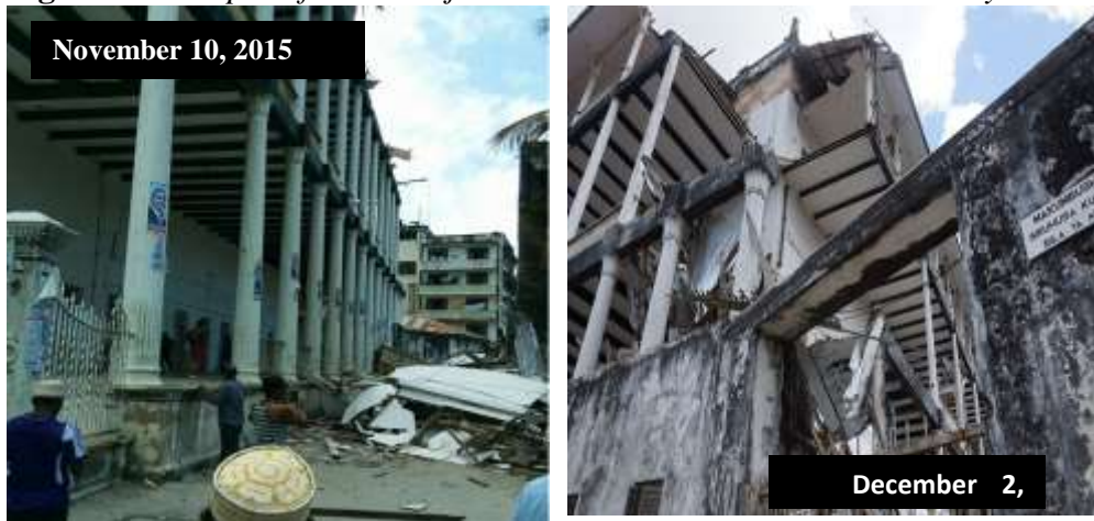
Figure 1. Collapse of Beit Al Ajaib Due Poor Maintenance and Heavy Rains
